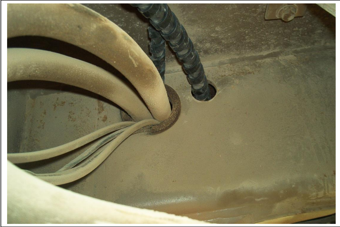
A/C hose runs along same direction as heater hoses.
